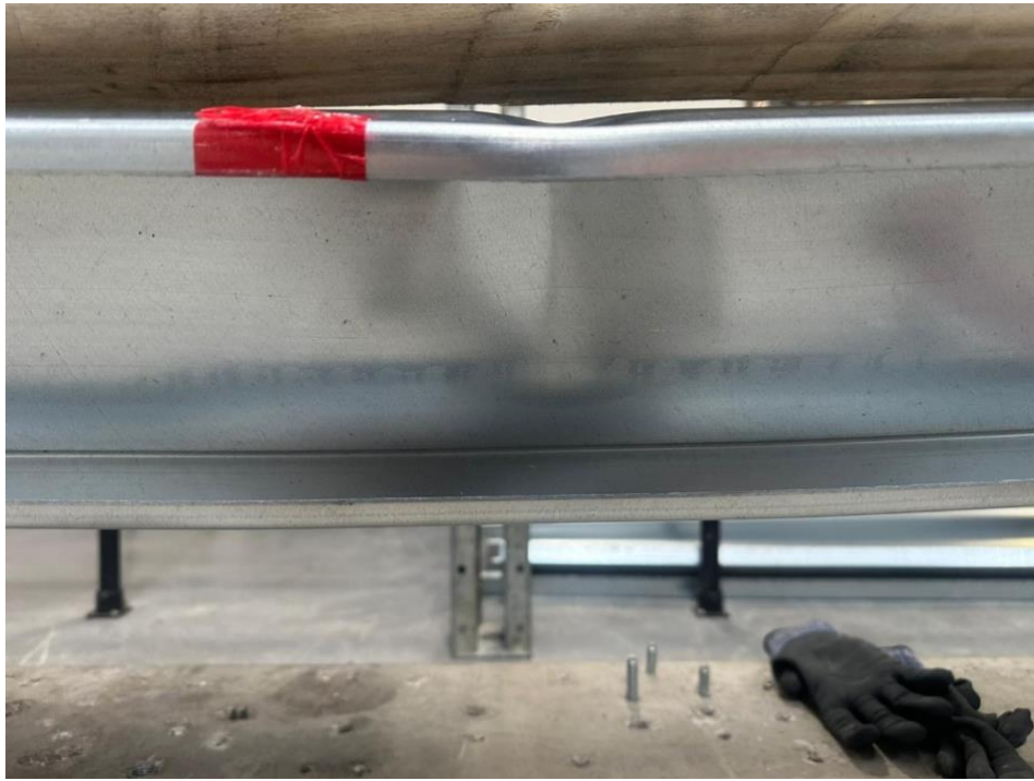
Figure 1 – C Perlin Failure
