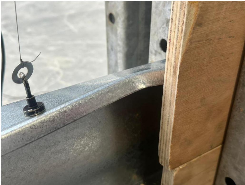
Figure 3 – C Perlin Failure
