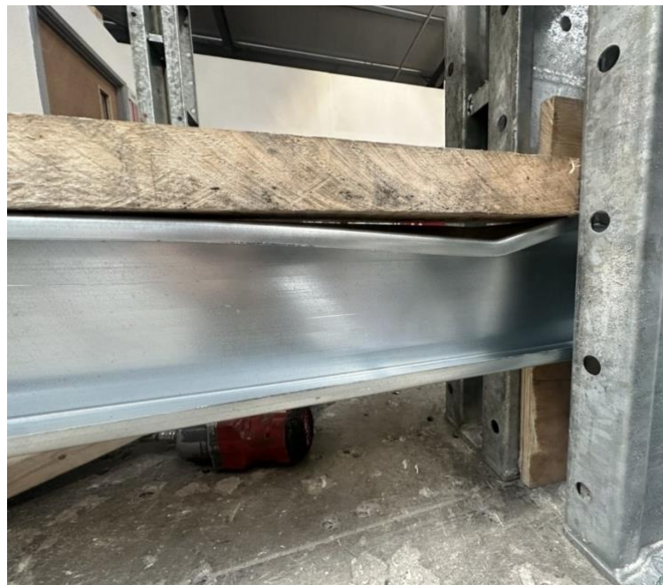
Figure 2 – Z Perlin Failure
