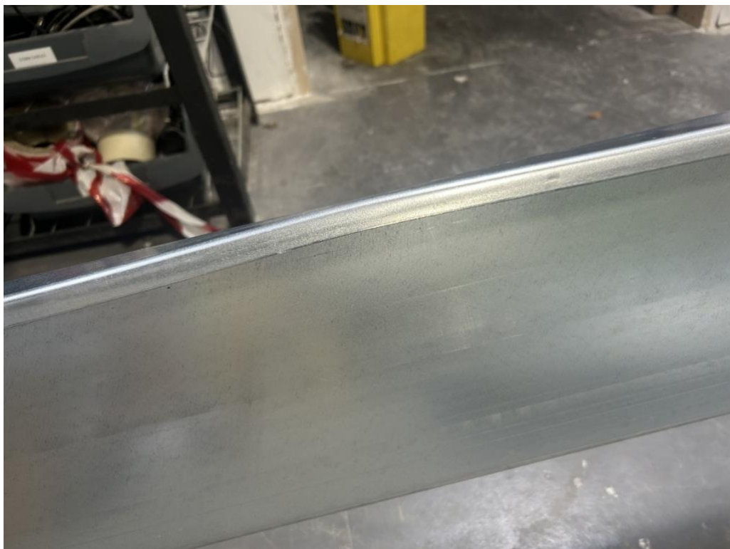
Figure 4 – Z Perlin Failure
