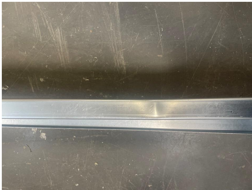
Figure 6 – Z Purlin Failure
